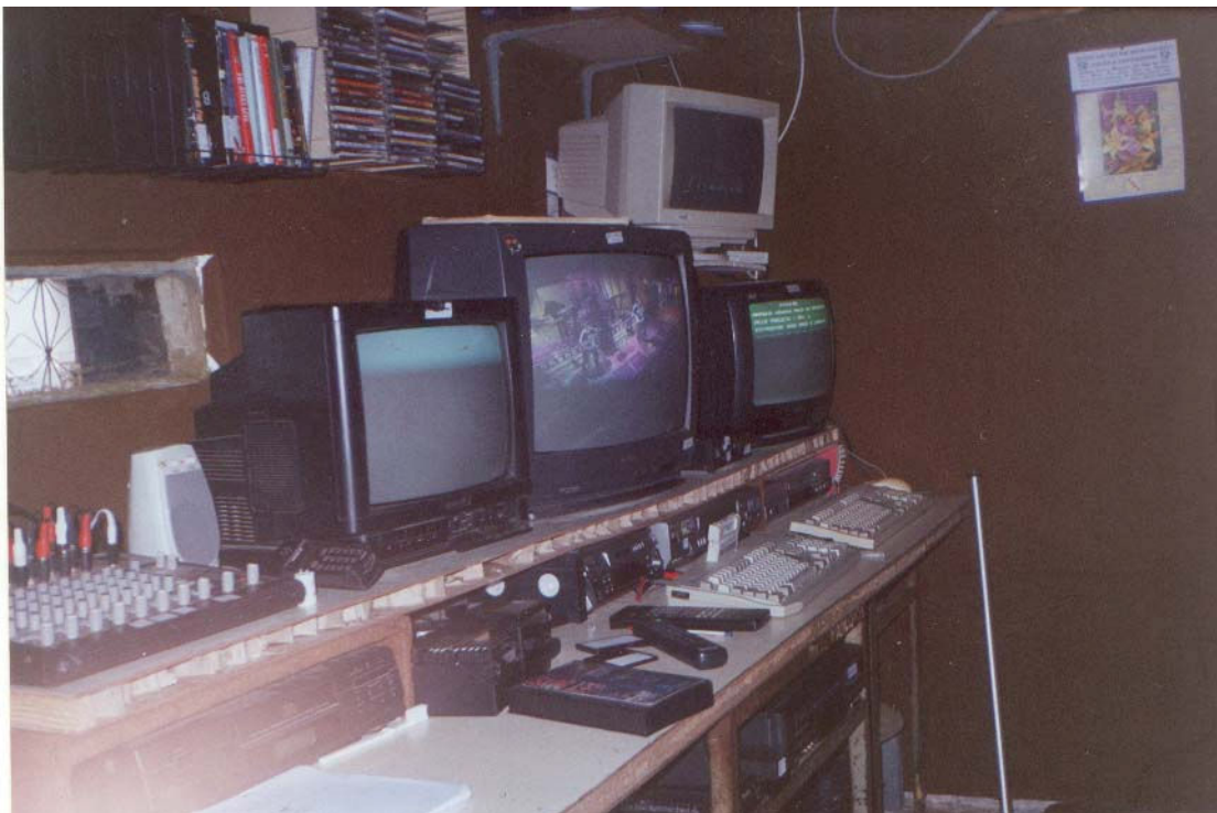
Sala de controle – ZSTV
